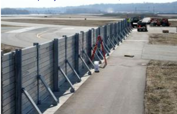
Temporary Floodwall - St. Paul, Minnesota
