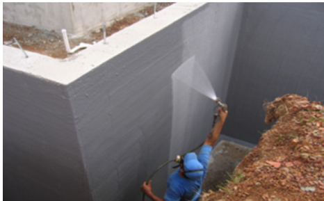
Spray-On Waterproof Membrane used for Dry Floodproofing
