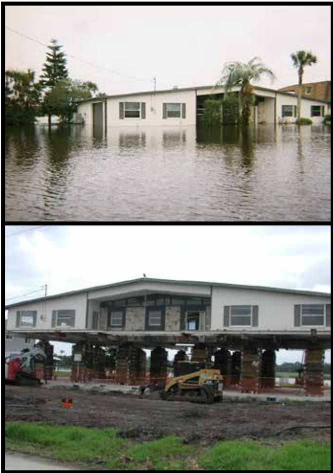
Structure flooded by Tropical Storm Fay and mitigation of the same structure in progress (photos courtesy of Volusia County)
