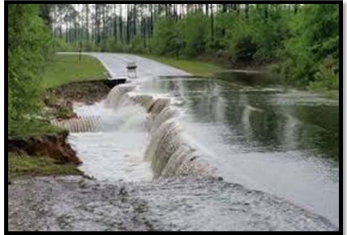
Roadway crumbles along CR3280 at Magnolia Lodge Road in Freeport. Photo courtesy of Walton County Sheriff's Office
