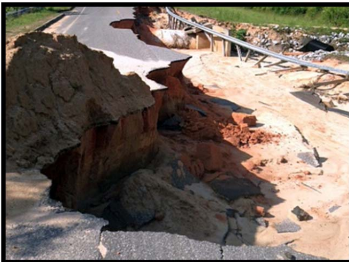
Road washed out due to flooding In Okaloosa County. Source: Crestview Bulletin, Matthew Brown
