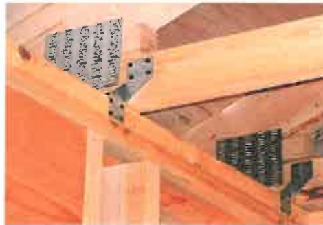
Hurricane straps are important to prevent roof lifting.
