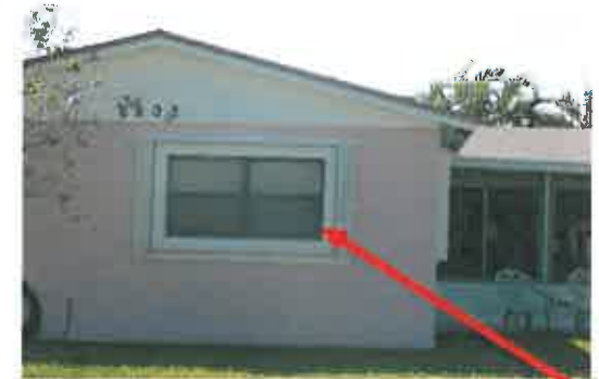
This home was disqualified for a discount because every opening except this window was protected with an impact resistant product.
