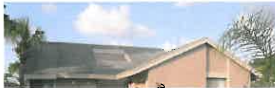
Every opening, including sky lights and gable vents, must be protected in order to receive the "Hurricane" rating.
