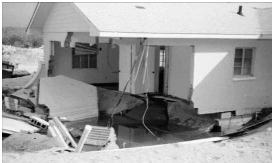
Figure 1-5 Beach erosion threatens tens of thousands of structures on barrier islands along the Atlantic Coast.
