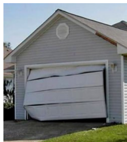
Garage door pulled out by the wind
