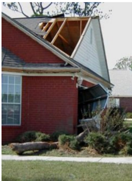
The failure of this garage door probably contributed to the loss of roof sheathing
