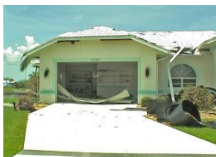
Garage door pushed in by the wind
