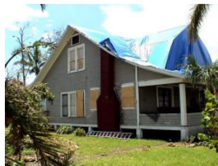
Tarps and plastic can be difficult and dangerous to install - note the boards holding down the edges of the tarps
