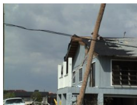
Temporary repairs to reseal the edge of this roof that lost the porch overhang as well as roof cover on the main part of the roof
