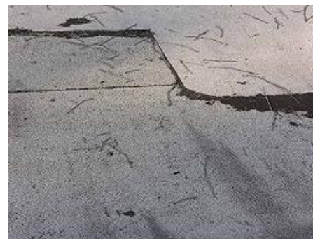
Patch on a section of membrane roof (click image for larger version)
