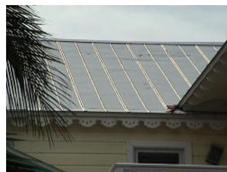
Holes in metal roof caused by the impact of flying debris (clay tiles in this case)
