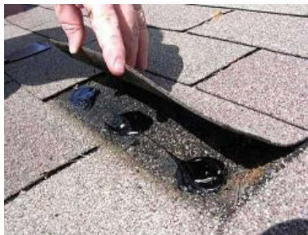
Applying dabs of asphalt adhesive under shingle tab (click image for larger version)
