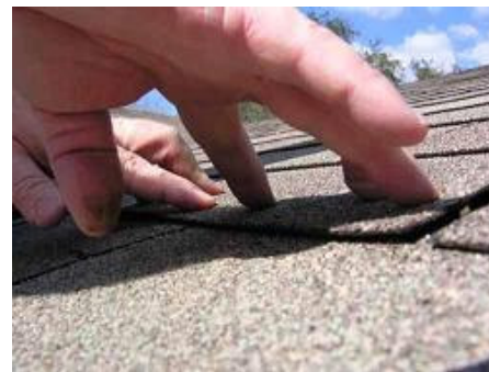
Pressing tab back against roof after applying dabs of asphalt adhesive (click image for larger version)
