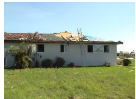
Temporary protection after storm damage to roof
