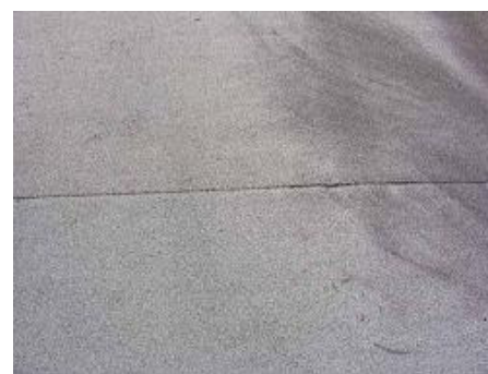
Portion of membrane roof showing seam between membrane sections (click image for larger version)
