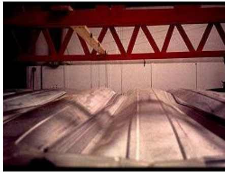
Standing-seam metal roof panels bowed up under about 30 pounds per square foot pressure applied to the bottom of the panels.
