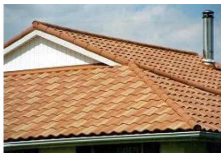
Metal roof made to look like tile (click image for larger version)
