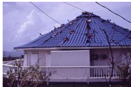
Typical hurricane damage to metal tile roof
