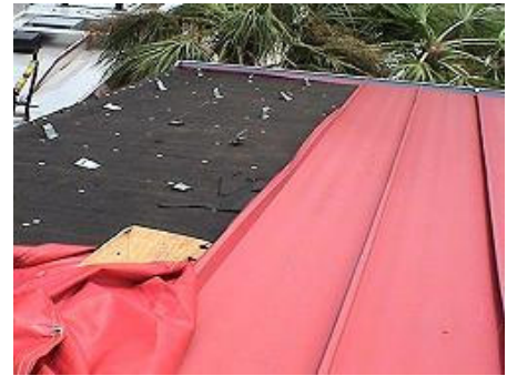
Standing-seam metal roof with missing panels. Note shiny clips that are curled into the seam between the metal panels
