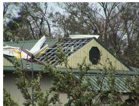
Metal roof without deck. When the metal lifts off, the interior of the building is exposed
