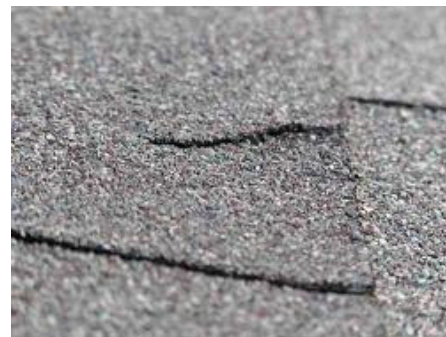
Cracked Shingle Tab
