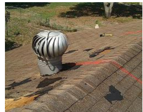
Roof Ventilation Turbine
