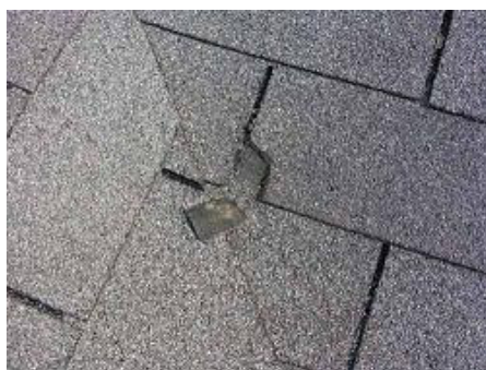
Broken Shingle Tab
