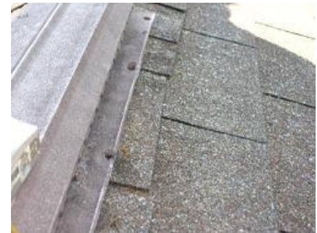
Ridge Vent Connection to Roof with Nails Working Their Way Out
