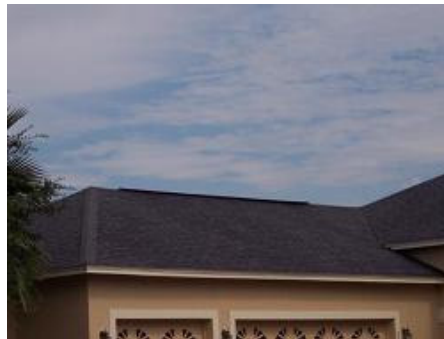
Ridge Vent on Shingle Roof
