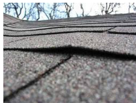
Buckled Shingle Tab
