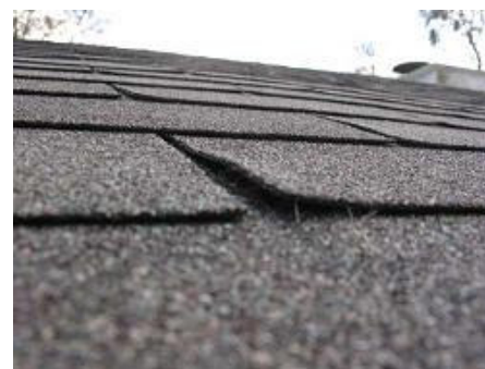
Partially Lifted Shingle Tab
