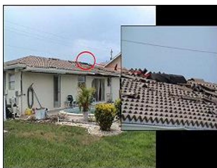
Off-ridge vents on tile roof house. The covered vent broke loose and allowed a tremendous amount of water to enter the house
