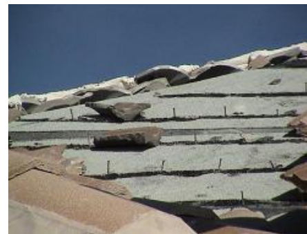
Mechanically attached tile - most of the tile failure was probably caused by impact of tile from a neighbor's house, but in some cases there were indications that the tile worked its way off the head of the fastener
