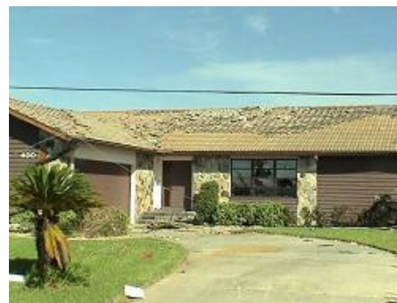
Windows broken by windborne debris
