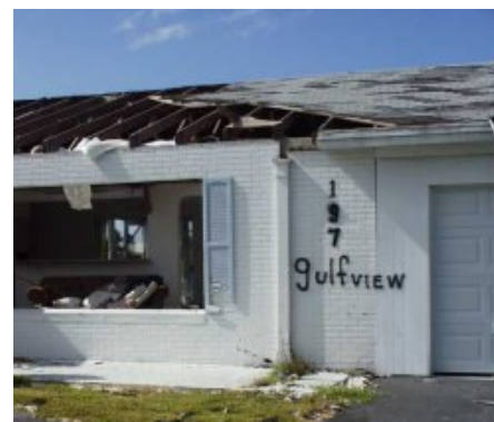
The roof over this porch lifted off and opened up the main roof and the house to the fury of the storm
