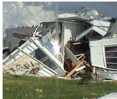
Storage shed blown apart by Hurricane Charley - note the tools still hanging on what is left of the wall
