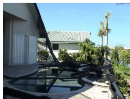
This used to be a nice screen pool enclosure before the hurricane blew through
