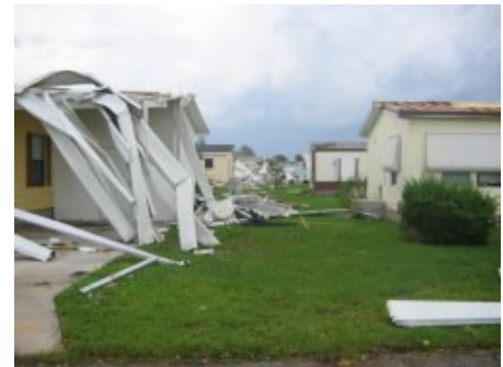
Metal panels on carport roofs frequently break loose in strong winds
