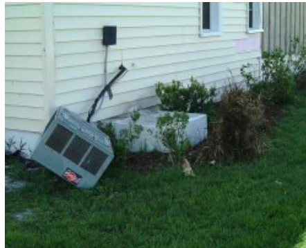
A couple of angle brackets could have kept this compressor in place
