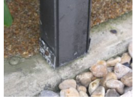
This column is held down by two rusty tech screws
