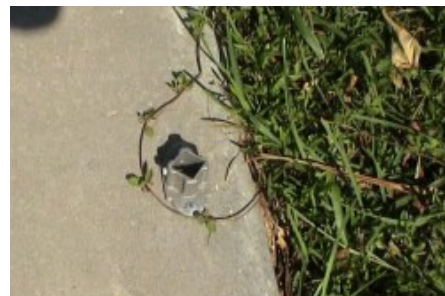
This cast aluminum insert once held a carport column in place - Imagine trying to hold down hundreds of pounds of uplift with the one tech screw on the left side
