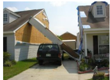
This chimney box was only attached with a couple of toe-nails near the roof
