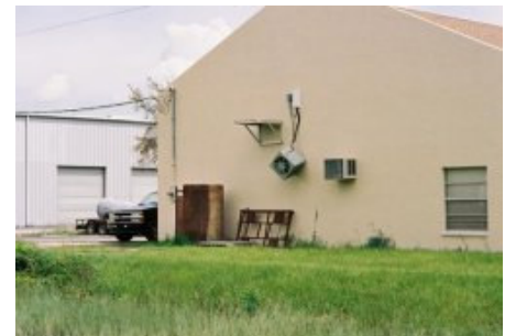
It would be nice to attach the equipment to the shelf
