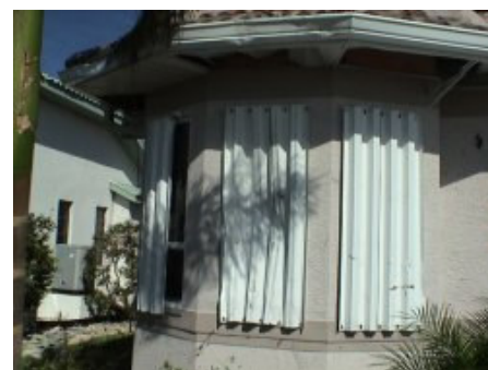
Tiles from surrounding roofs banged up these shutters
