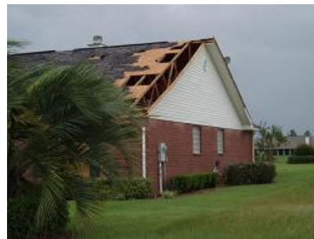
Roof sheathing loss at gable end. This is a common failure point.
