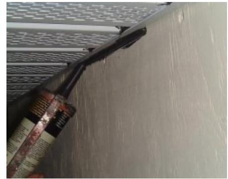
Caulking bottom edge of soffit wall J track to wall to improve anchorage of track - black caulk shown for contrast.
