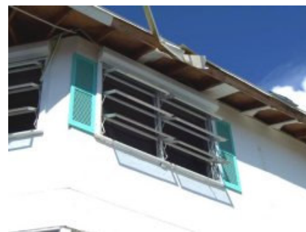
Soffit damage was widespread - this photo shows both fascia cover and wall track damage
