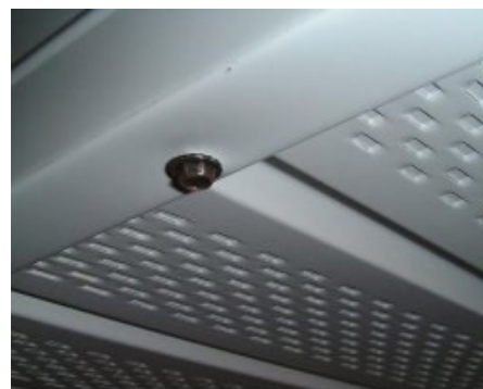
Screw inserted through edge of fascia cover, through soffit panels and into fascia board
