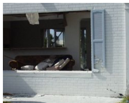
This window and frame was pushed in by the wind
