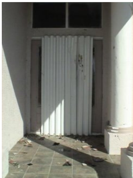
This shutter took a direct impact of a large tile missile. The door behind the shutter was damaged as a result.
