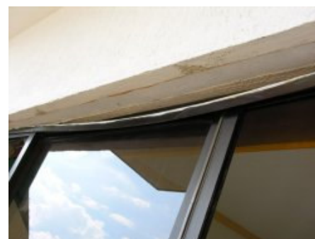
A track anchorage failure for a set of sliding glass doors. Note the single fastener hole above the door panel.
