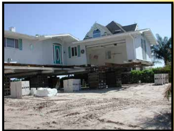
The average cost per structure elevated was about $265,000 for projects included in this assessment (photo courtesy of Volusia County, Florida)
