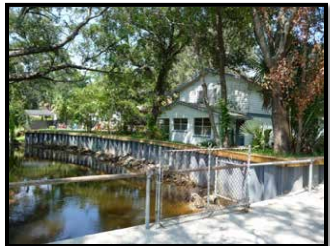
Post-mitigation image of project site for FMA-PJ-04-FL-2008-001 (photo courtesy of City of Jacksonville).
