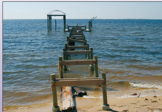
Destroyed dock from high seawater and winds
