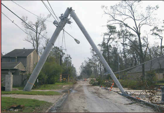
Destroyed concrete utility pole with light fixtures
