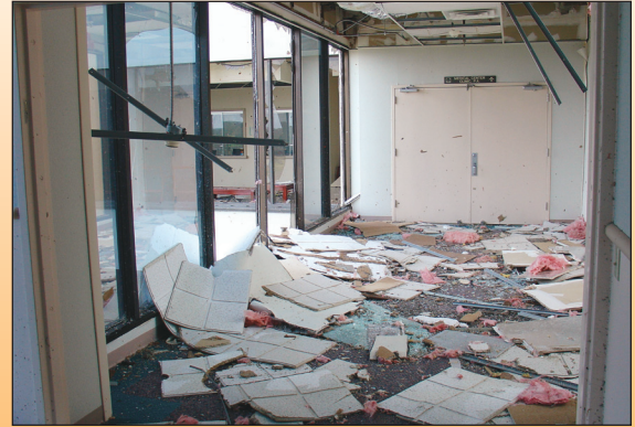
Interior damage of a building from Hurricane Ivan
