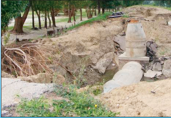
Damaged levee caused by floodwaters
