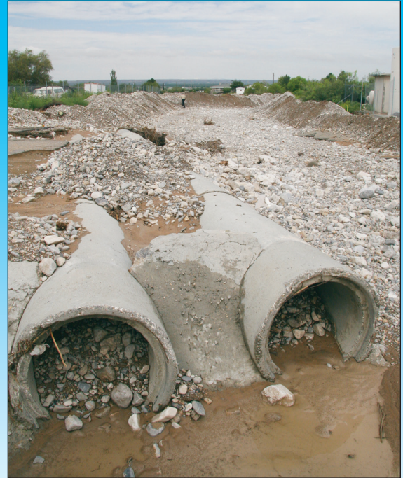
Clogged drainpipes as a result of flooding
