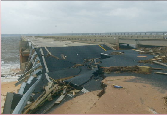
Bridge destroyed as a result of Hurricane Ivan
