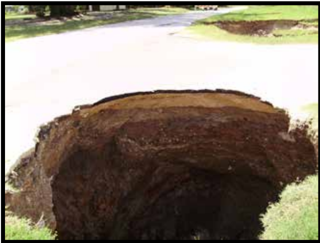
Local partners were able to provide photographs of Tropical Storm Debby's impact, such as this sinkhole, along with personal knowledge of project performance (photo courtesy of City of Live Oak).
