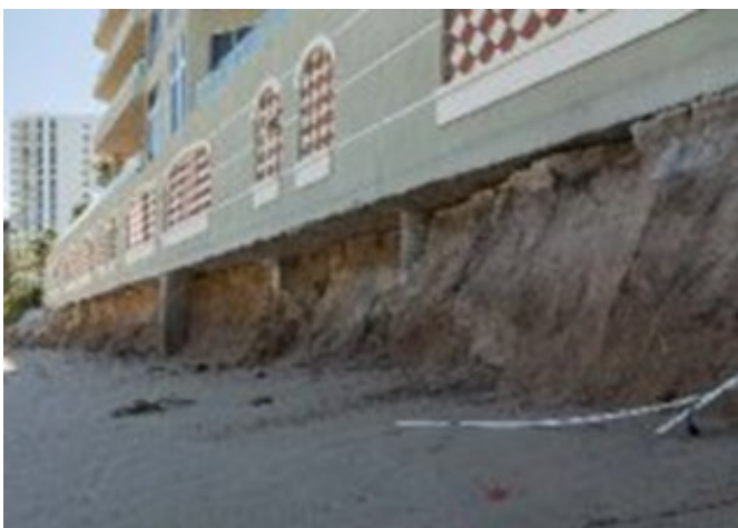
In this October 2012 photo sand has been pulled away from the beachfront of Ocean's Edge by high surf.
