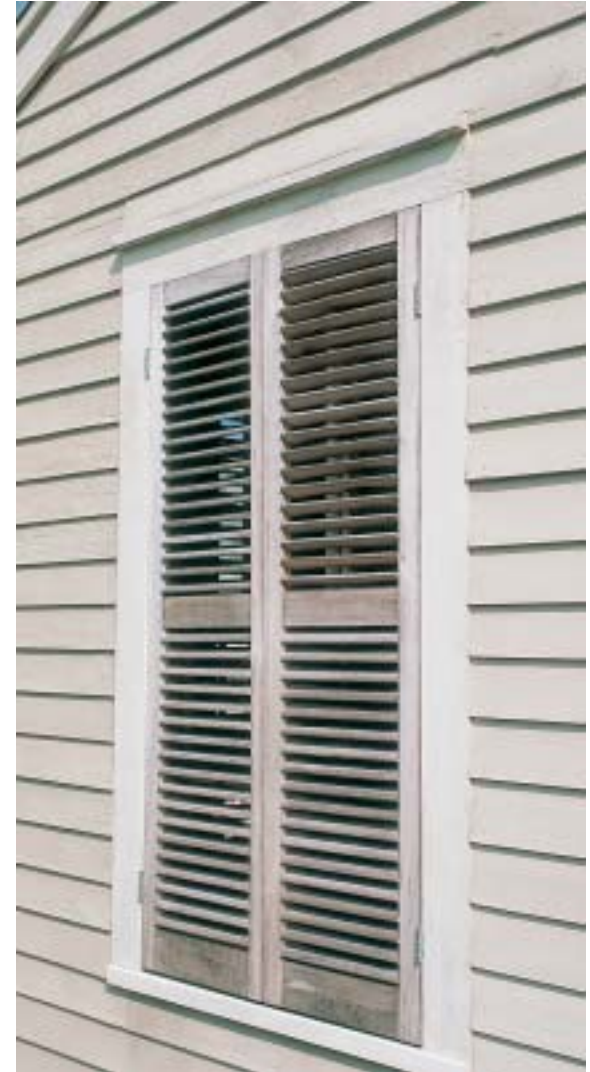
Historically, some buildings had shutters to protect them from storms. VIVIAN YOUNG
