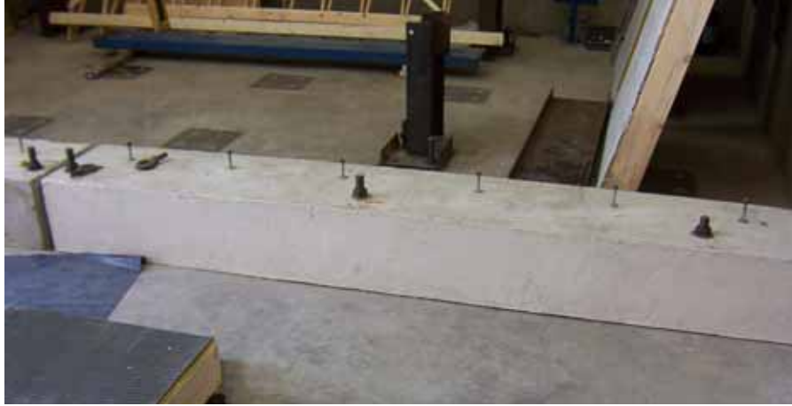
Figure 3.3: Close-up of Concrete Foundation Block with J-Bolts and Threaded Rod
